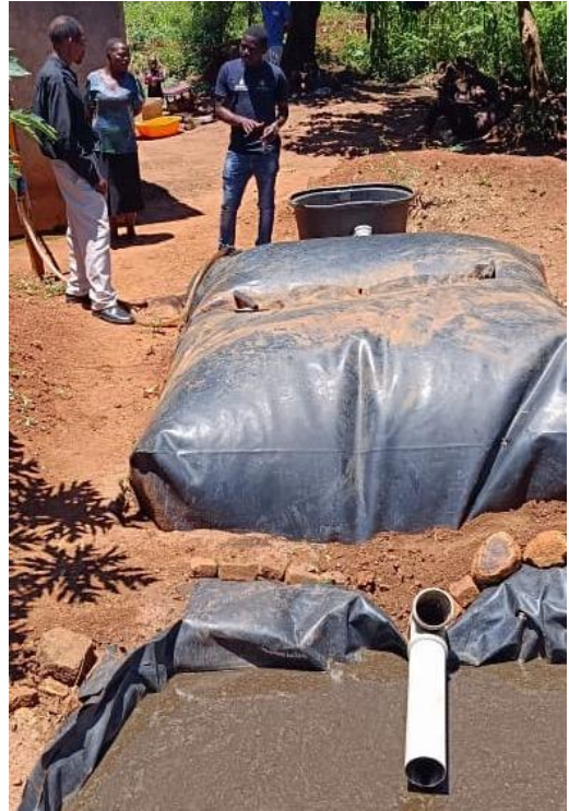
Photo: A biodigester installed at an EcoGen client's home. Credit: The Canopy Lab
